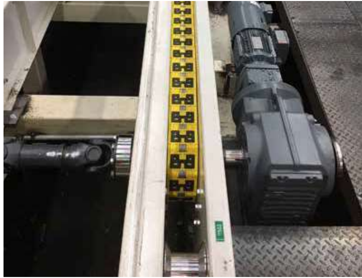
Conveyor equipped with Rexnord 3125 HYB 12 Series MatTop Chain.
