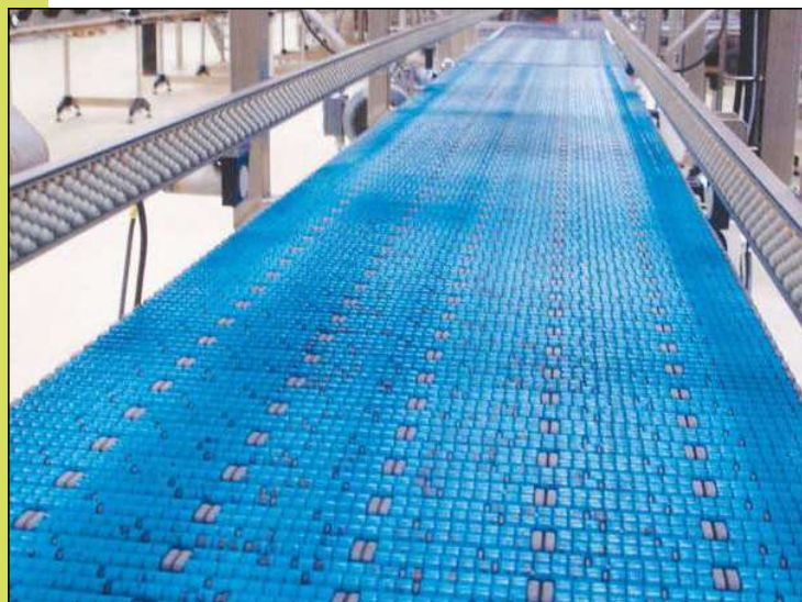
CONVEYOR FOR TRAYS WITH CANS.
